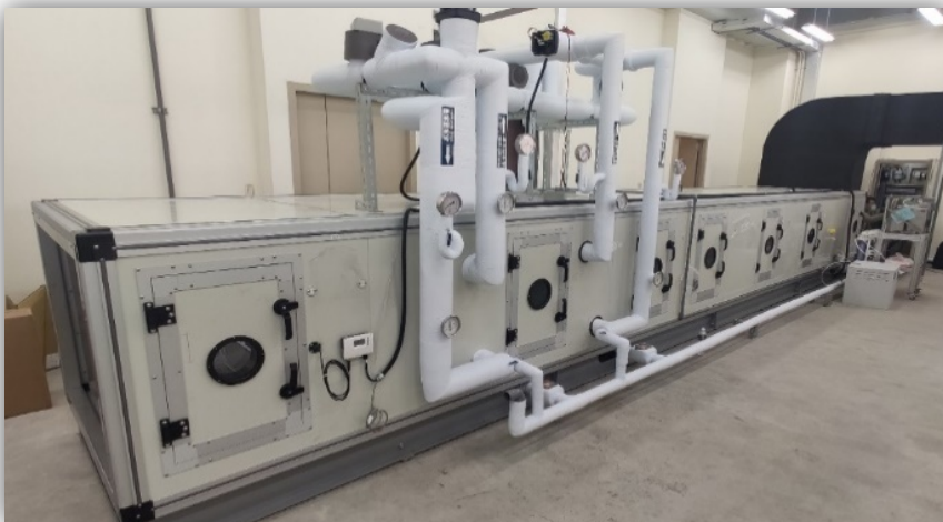
Full Scale Chemical Filter Test Rig.
