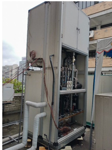
Water chiller with integrated cooling tower
